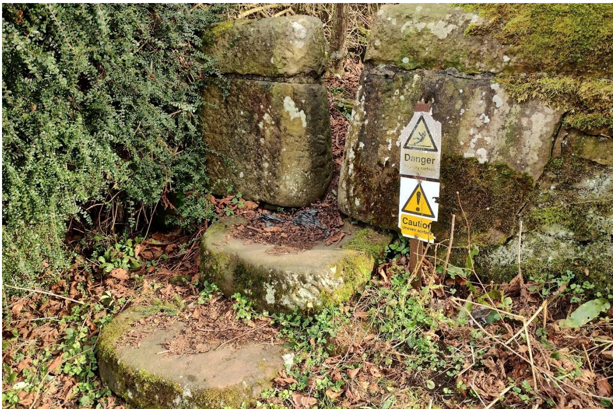
Figure 16: Boundary wall to footpath with worn steps
